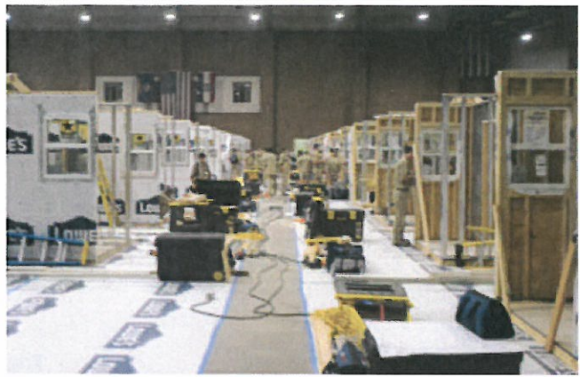
At 10:15, there was a mandatory break, and the competitors got a quick clinic on installing windows.
